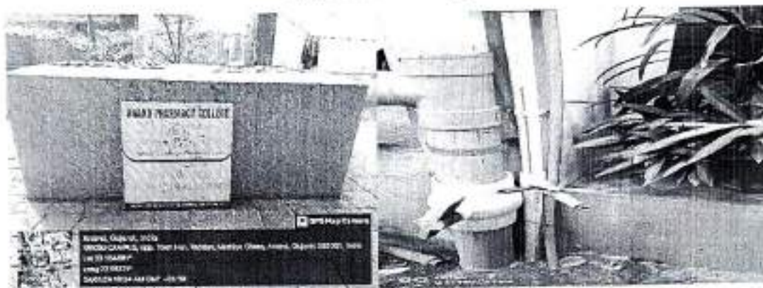
Rain water Harvesting Plant
